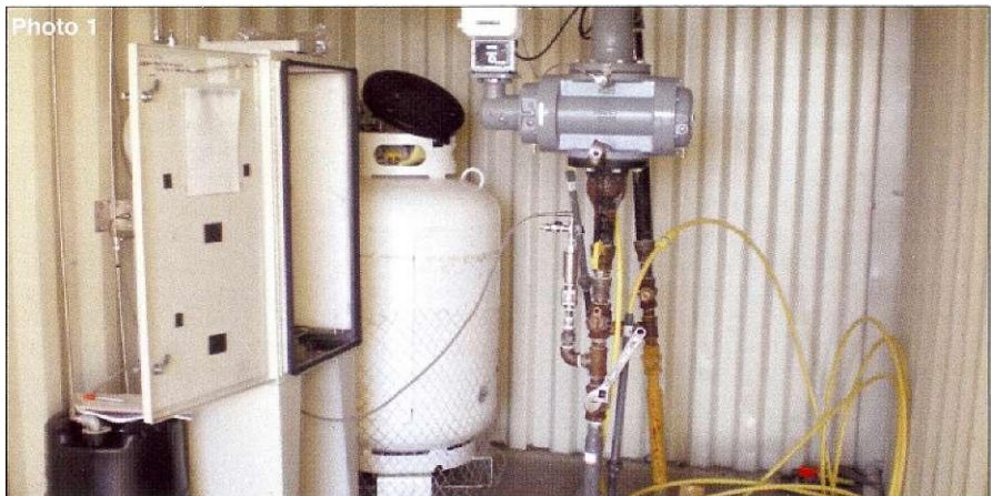
Photo 1: Set-up of Temporary Odorant Injection System. A rented marine container was installed with a hole in the floor to give access to the risers at the beginning of the new underground gas line. A flowmeter and pressure gauges were installed to be able to calculate retention time to the tail-end of the pipe and to keep track of the volume of gas flared during the pickling process. A rented YZ injection system was installed (white cabinet) along with an odorant cylinder (white cylinder) and a scrubber for mercaptan vapors from the injection system (black drum)
