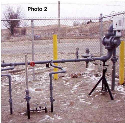
▲Photo 2: Bypass Odorizer. At the same site where the marine container stood months before, a King-Tool 3-B bypass odorizer was installed to compensate for odor fade still occurring in the new line. The odorizer is buried underground to minimize temperature variations of the liquid odorant and prevent it from boiling off. Only the level gauge, test ports and needle control valve remain above ground. The red handle seen on the main line is that of the gate valve which controls how much of the gas flow is diverted to the bypass.
